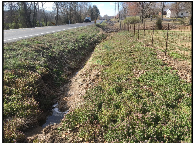
Figure 4: Narrow Shoulders and Steep Drop-offs into Excised Ditches
