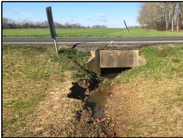
Figure 5: Steep Drop-offs at Culverts
